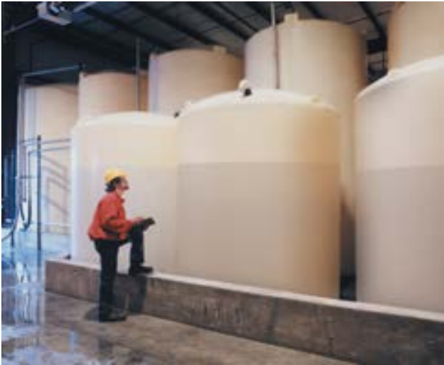
Assmann polyethylene vertical storage tanks at a northern Illinois chemical company.
